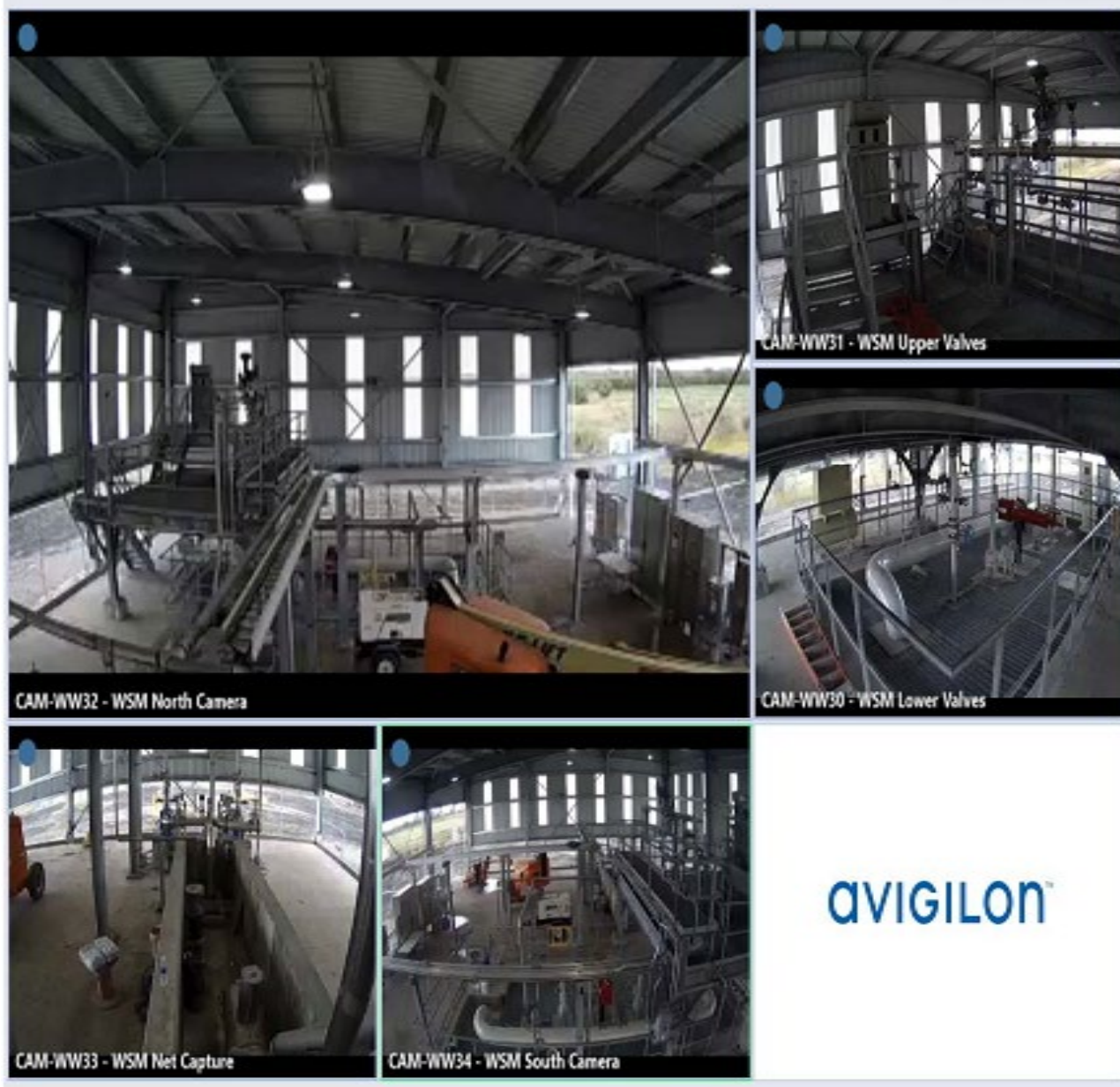
Photograph M View from WSM During Construction Cameras of the WSM December 30, 2020
