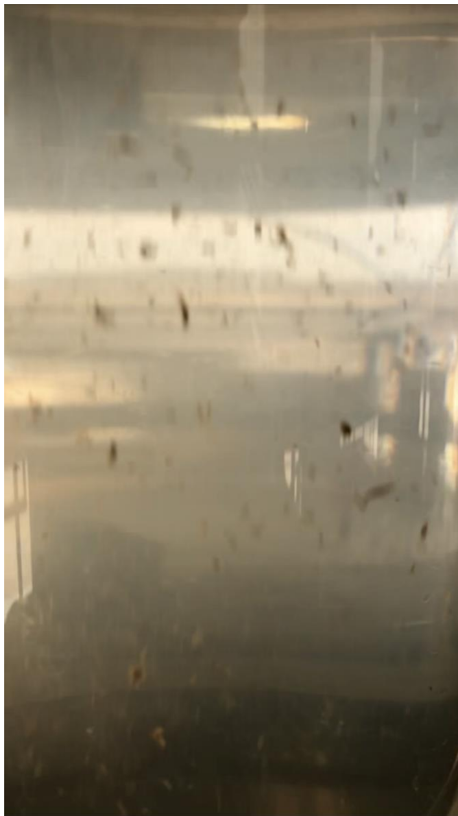
FIGURE 46 - UNACCEPTABLE PRESENCE OF SOLIDS IN SIGHT GLASS (CLOSE UP VIEW), TRIGGERING A MANUAL SAMPLE
