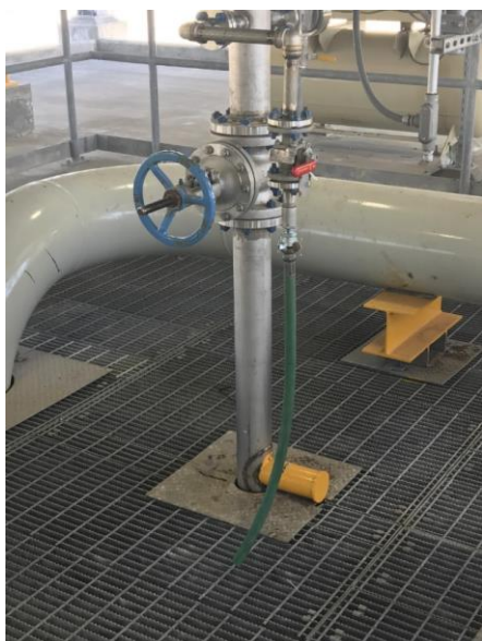
FIGURE 28 – MANUAL VALVE ON FIRST FLOOR
