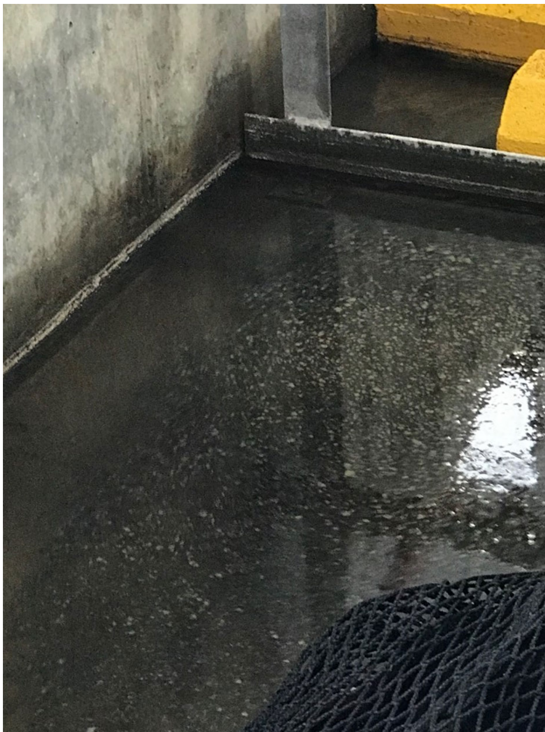
Photograph H Plastics floating in Concrete “Bathtub” June 30, 2021
