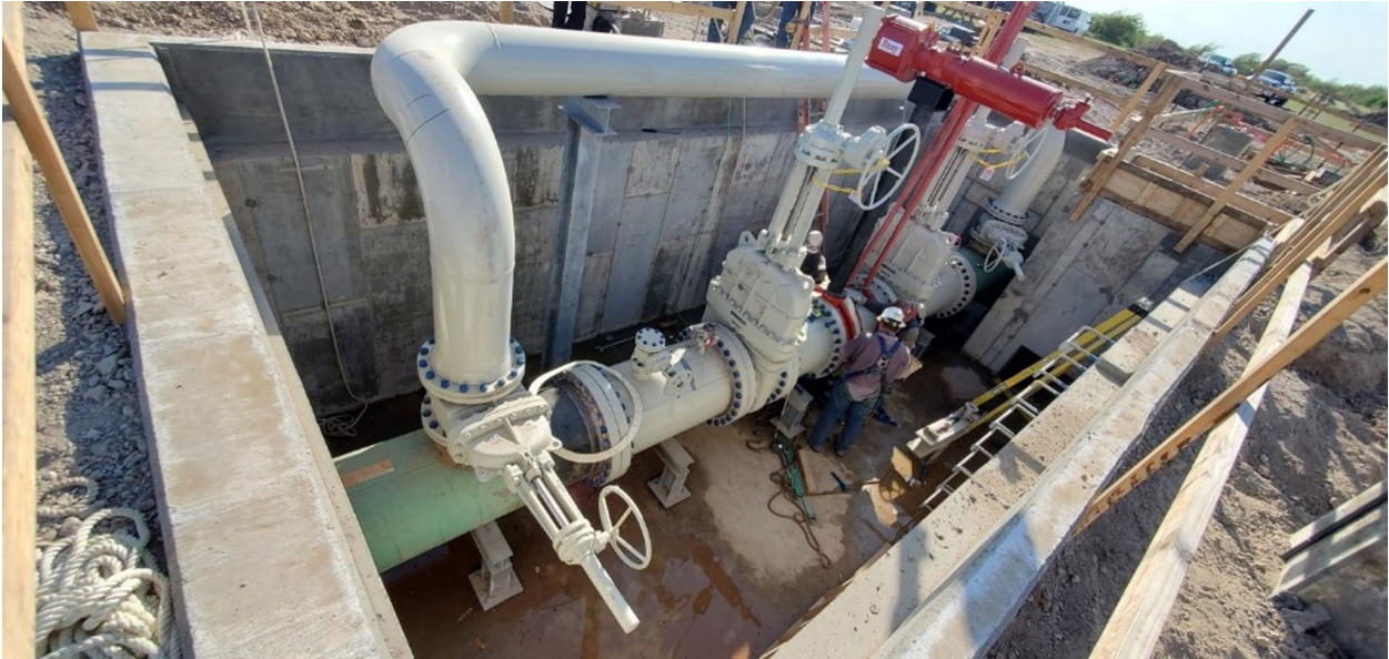
Photograph E 30-in Outfall line and Sampling valves and pipes to the WSM October 15, 2020
