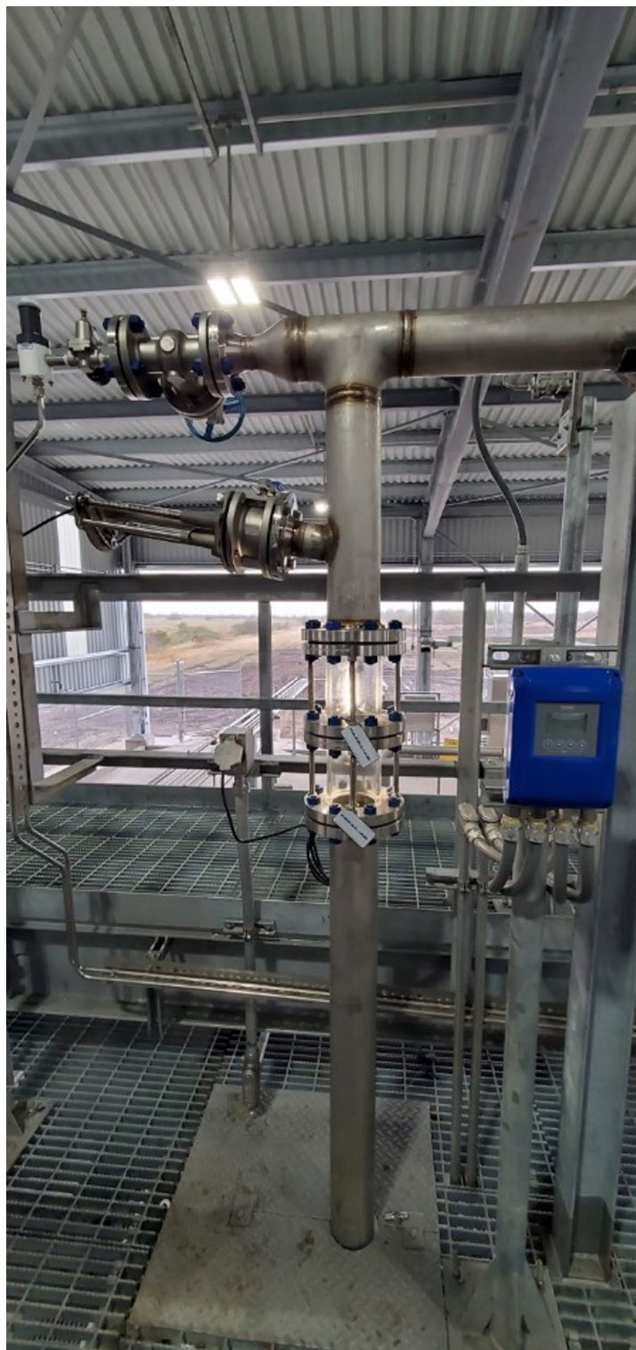
Photograph L Sight Glass at the WSM December 30, 2020
