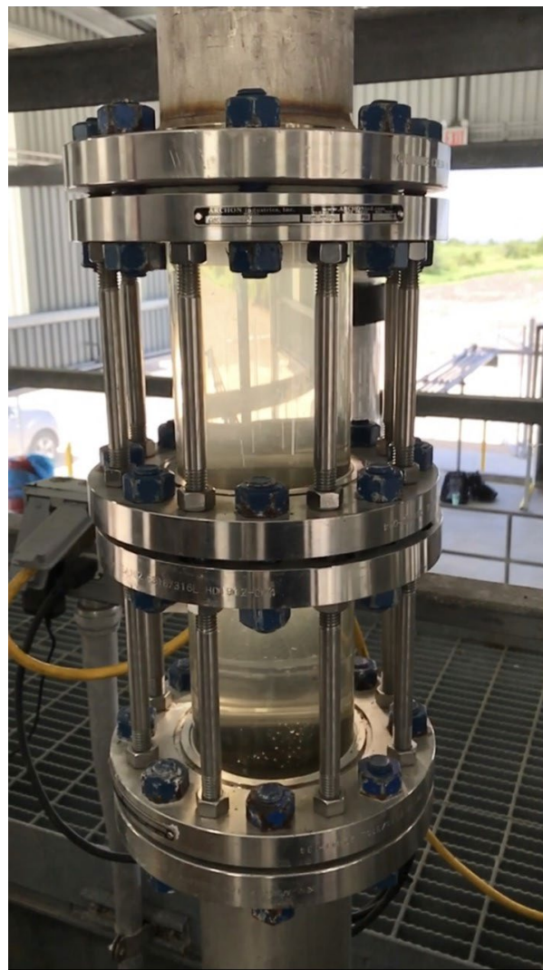
Photograph K Sight Glass at the WSM with Flow August 20, 2021
