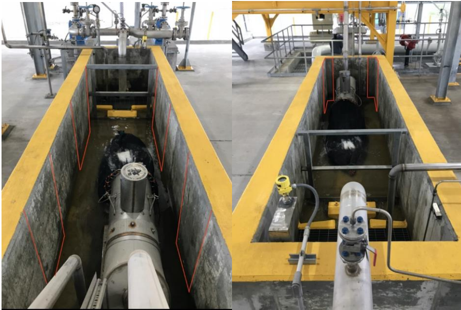
FIGURES 59.1 AND 59.2 – REDLINE MARKS TO BE INSPECTED FOR POWDER WITHIN SUMP AREA
