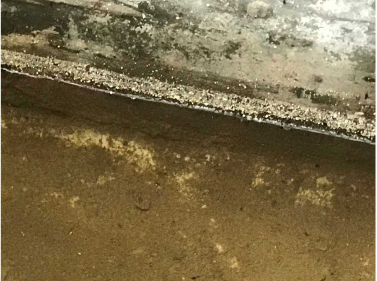
Photograph I Plastics floating in Concrete “Bathtub” June 4, 2021
