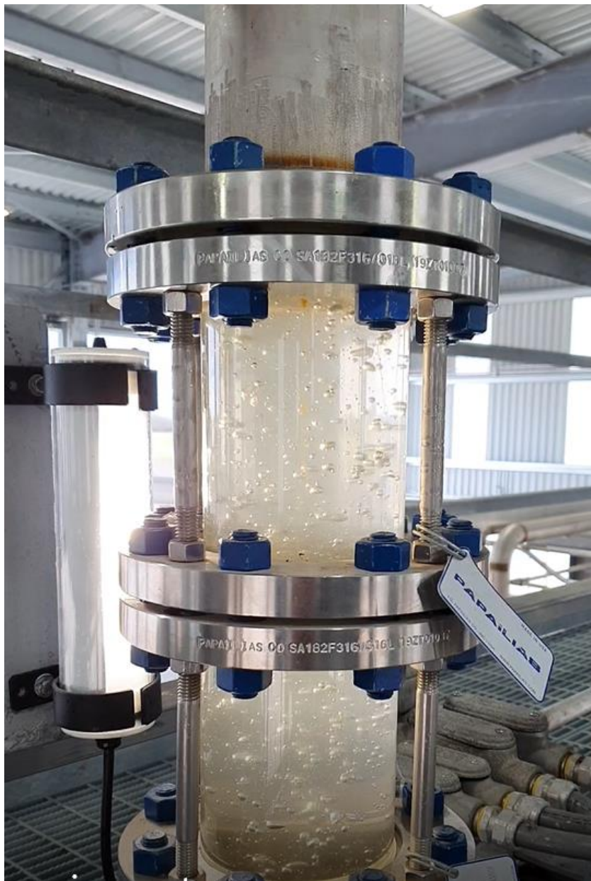
FIGURE 43– UNACCEPTABLE PRESENCE F BUBBLES IN SIGHT GLASS WOULD INTERFERE WITH TSS READINGS
